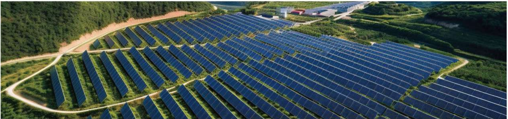
Location: South Africa Capacity:750kW/1.5MWh
